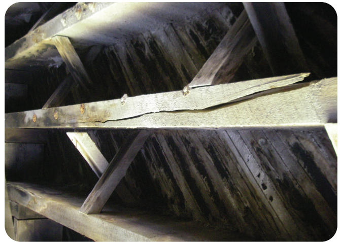
Image 2. Cracked Girder (D-28-P)
