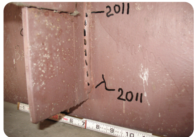
Image 4. Fatigue Crack (E-16-LT/LU)
